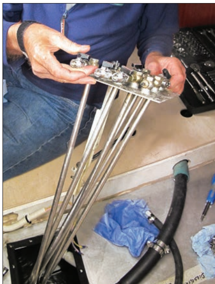
The author gains excellent access to his tank by pulling off the plate holding all the fuel suction and return lines, including his fuel tank sampling line.
