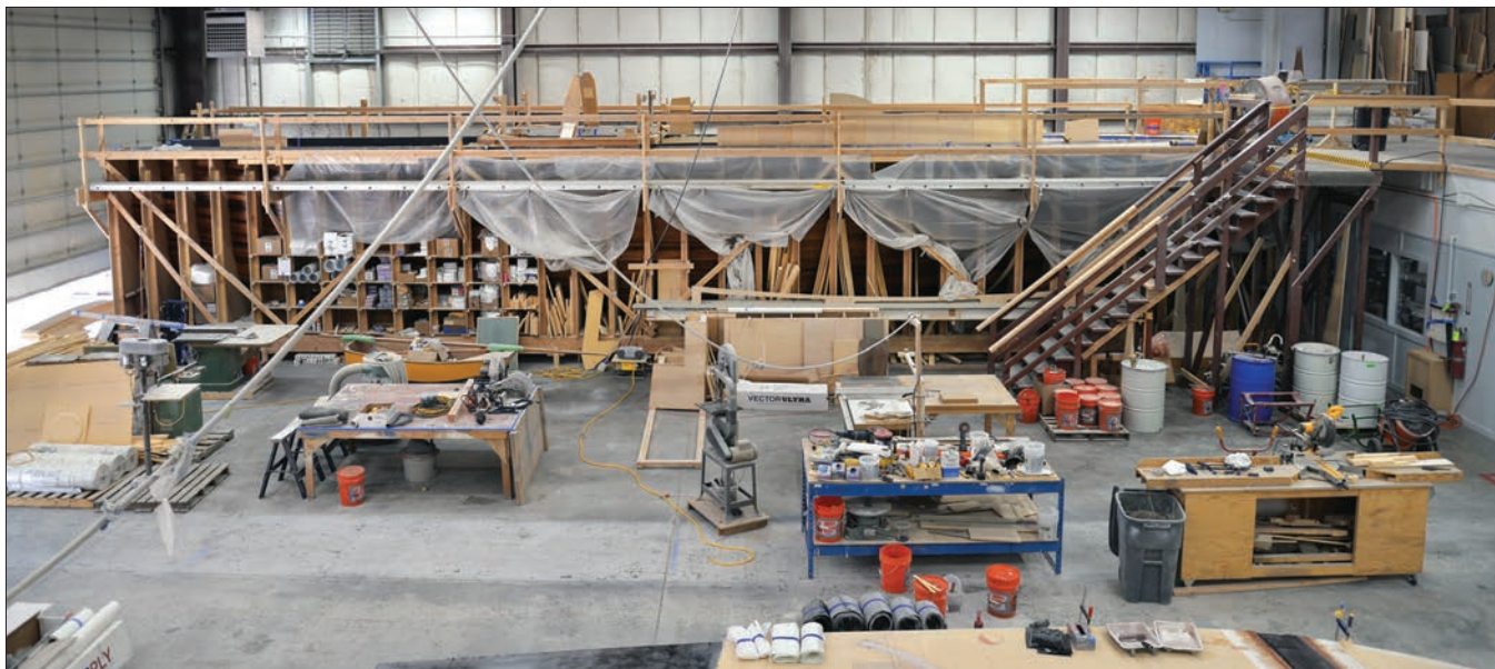
This view from atop the first catamaran looks across the shop floor at the hull mold. Note temporary storage between stations of the mold.
